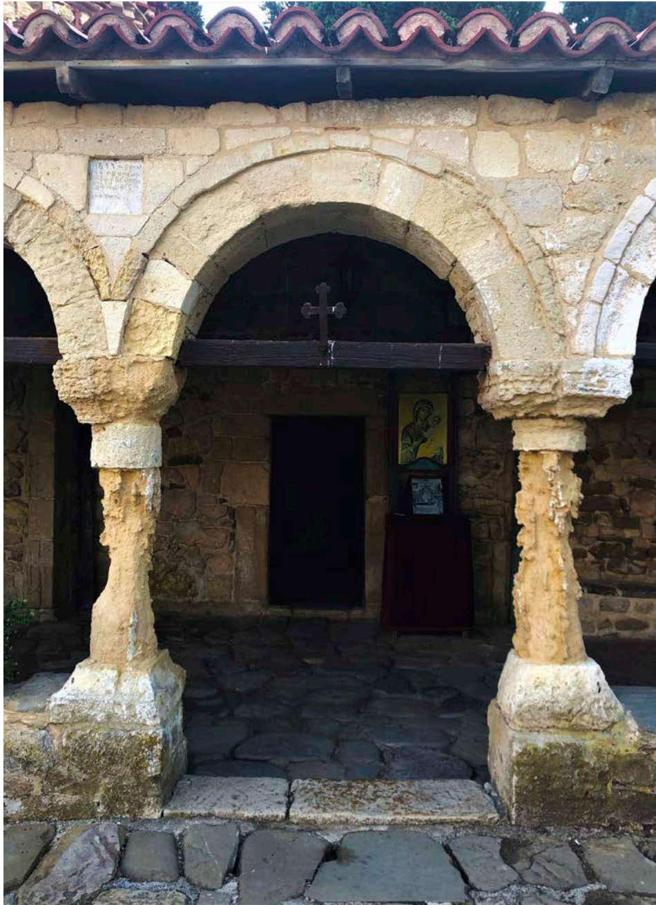
Figure III-5.11 The eroded columns of the portico as symbolic image of the church.
