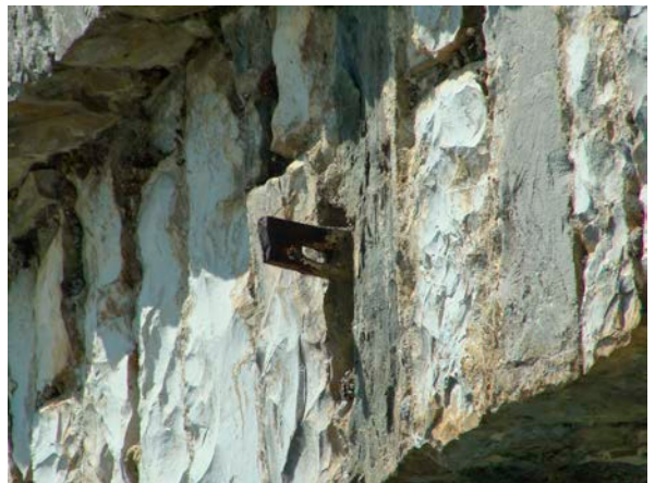
Figure I-5.1.5 – A detail of the head of a transverse steel tie rods lacking of wedge.
