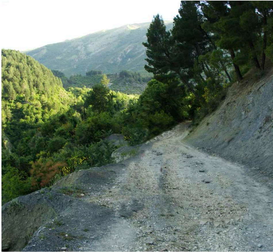
Figure I-4.3.10 The poor conditions of the road to Përmet make the life of the villagers difficult and hamper the tourism development possibilities.
